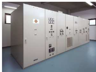
2 浄水場高圧設備 High-pressure water purification plant equipment 浄水厂高压设备
