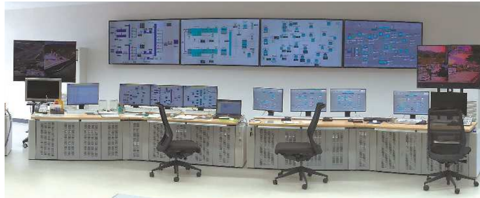
1 浄水場監視制御システム Water purification plant monitoring and control system 浄水厂监视控制系统
